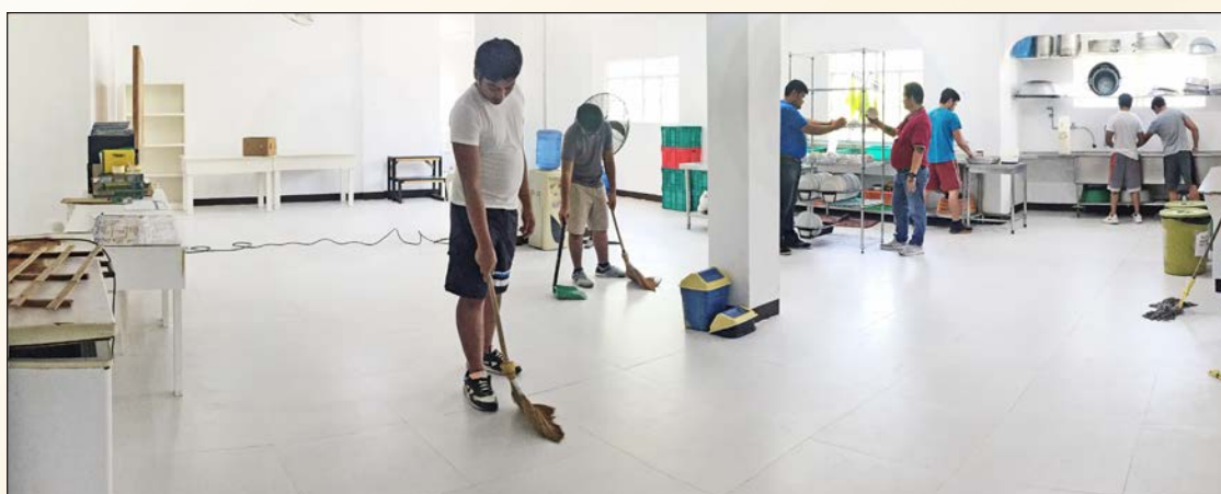
FACILITY UPGRADE — While the TC was taking refuge in the Blusyl Resort, SELF forged ahead with the project to refurbish the entire basement of the Multi-Purpose Hall that had been put on hold by the evacuation. With no residents around it was the opportune time to tear down nonessential rooms and retile the entire floor. Funds for this project had been earmarked from the proceeds of the 2019 Yuletide Show that raises funds to improve the facilities. In the photo, residents begin setting up the kitchen and the pantry in the handsomely renovated basement. More facility improvements are in scheduled in the coming weeks.
